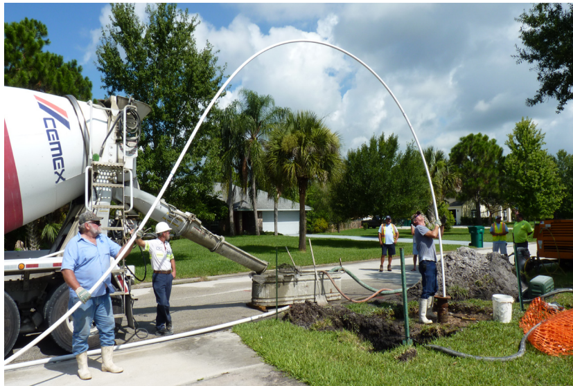
Workers lower a "tremie" into the well to pump in cement in order to plug the well.
