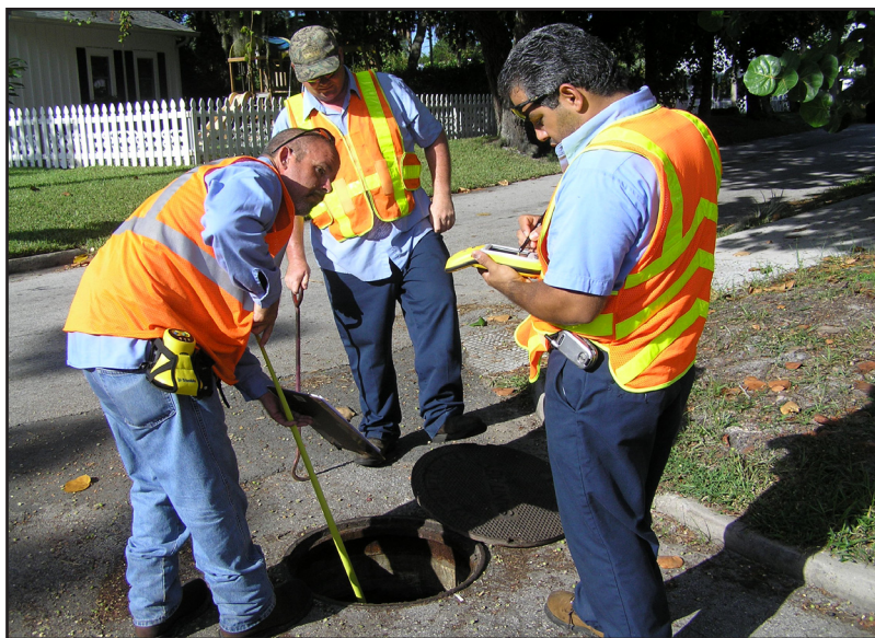
In the Olde Eau Gallie area recently, Butch Burke (left) measure manhole, while Rubin Rosado (right) enters data into the Trimble unit and Darrell Swain (back) prepares to replace cover. Others who will be assisting include Dana Christianson, James Jordan, and Robert Coger III.
