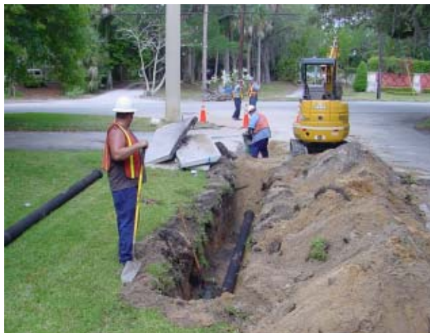
Installing new 6-inch line for one of the new fire hydrants as part of the project are Bernie Neanover (foreground) and Donnie Thompson. In the background are Foreman Tim Mulligan (right) and Dave Riley. Odell Wadlington and John Hummel were also part of the crew for the project.
