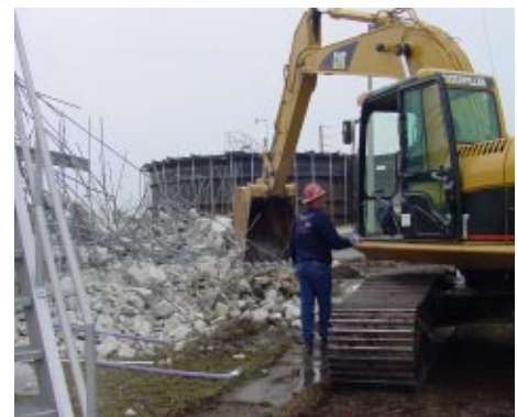
A trackhoe used in the demolition of one of the concrete tanks.
