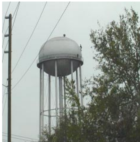
Two workers on top of the Wickham water tank prepare it for demolition.
