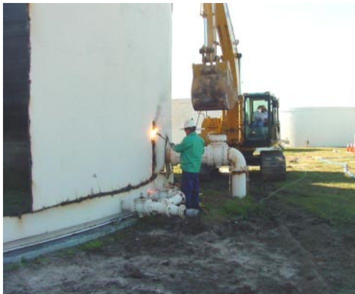
Worker with Cross Environmental Services uses a cutting torch to demolish one of the steel ring package treatment units.
