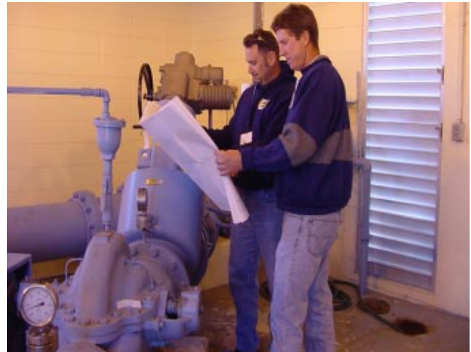
Bill Spann (left) and Electronics Technician Ray Elden go over plans for the valve replacements. One of the valves has already been replaced, with two more to go. The project should be complete by early April.
