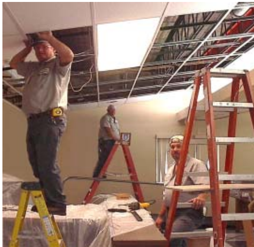
Performing prep work for the project are Don DeLoach (back on ladder), George Wood (front on ladder), and Dave Lindsay.
