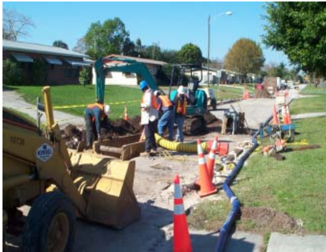
Workers from Instituform , the City's contractor for the project, begin pipe bursting procedure.
