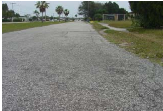
One of the roads to be resurfaced shows its poor condition.
