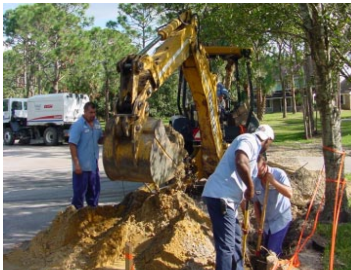
Crew completes finishing touches on Laguna Vista water line project. From left are Shannon Brogan, Robert "Colgate" Coger, Doug Effler, and Robert Sigman operating the backhoe.
