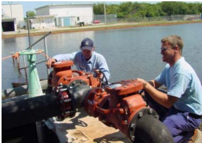
Art Townly (left) and Steve Clemons work on installing new backwash recycle pumps at the surface water treatment plant.
