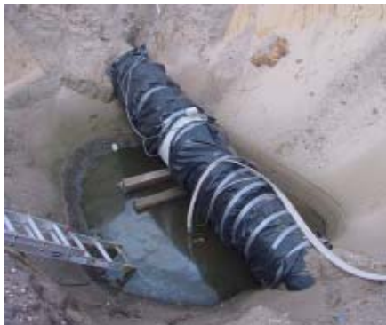
New flow meter is located in the center of the 24-inch effluent line.
