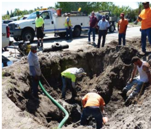
Workers with YCom work to remove an unexpected valve so the new HDPE pipe can proceed through its path, while City crews and staff, along with Karl Morrison from YCom (background, right, in bright orange shirt) observe.
