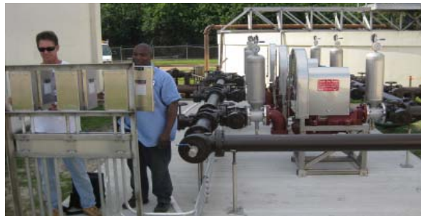
City Electricians Ray Eldon and David Cooks install the electrical service and controls for the new sludge filter press pump station.
