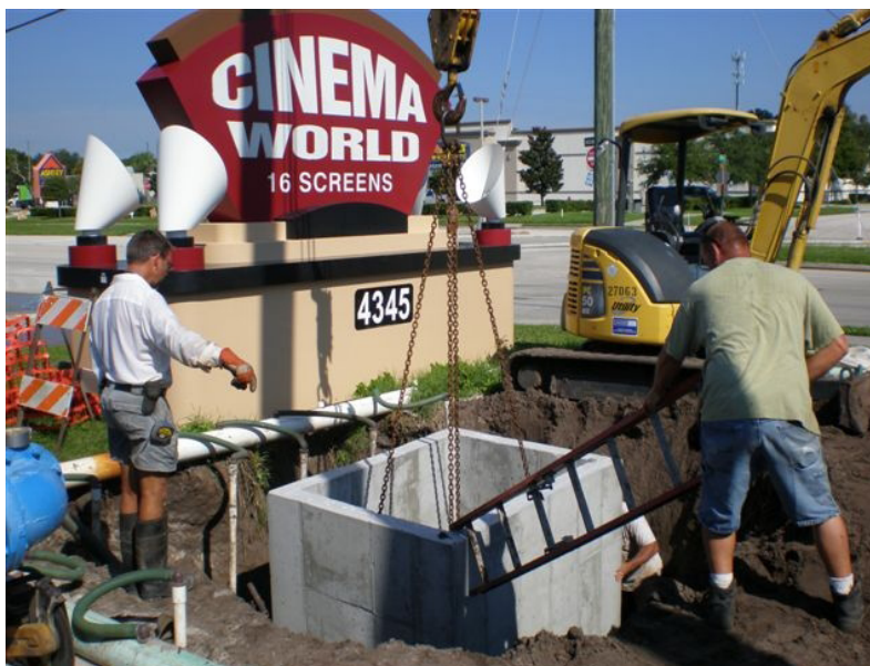
Workers from Maxwell Construction install valve vault for the pressure sustaining valve at the Cinema World location. The vault allows for maintenance access when needed.
