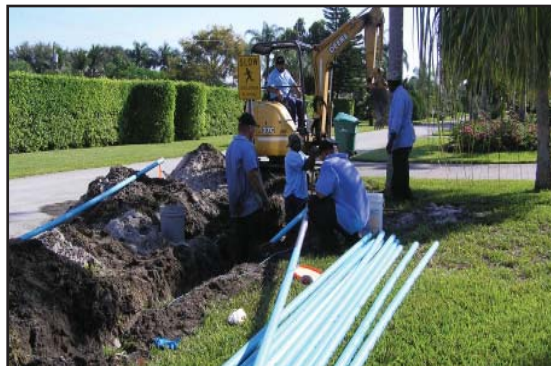
Equipment Operator Robert Sigman uses backhoe to dig trench. Pipe will be fed into casing. Crew includes Rob Smith (left), Skeet Phillips, Manny Parker, and Shannon Brogan.
