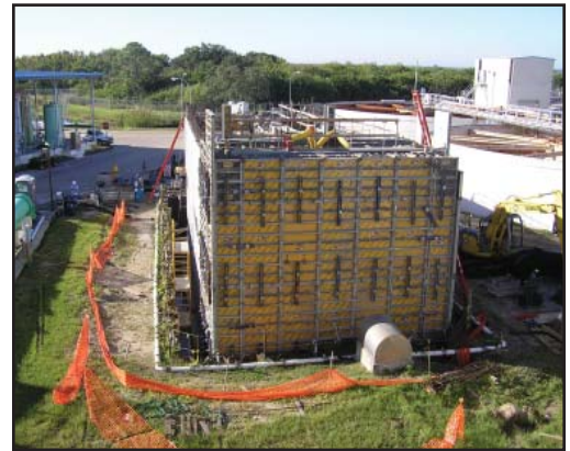
Ozone contactor basin.
