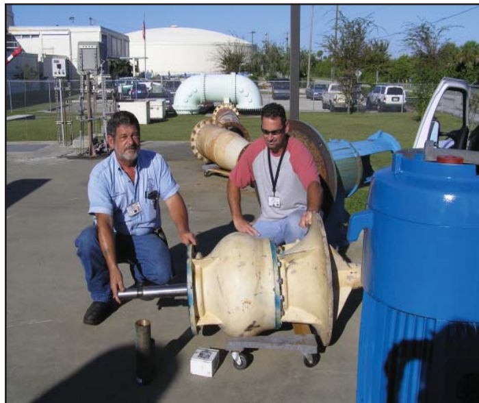
Maintenance Foreman Joe Dean (L) and Supervisor Bill Spann check lower pump-end bowl assembly.
