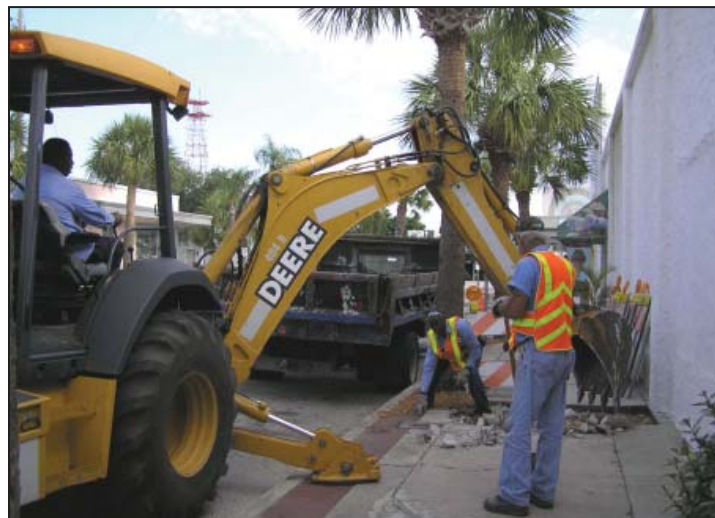
Manny Parker digs up section of concrete using the backhoe. Silas Scott pulls up pieces after he had jackhammered the area to loosen the concrete. James Post, standing, also worked on the repairs. Not pictured are John Clark and Al Slagle, who also were involved with the repairs, along with Foreman Joe Gervais.
