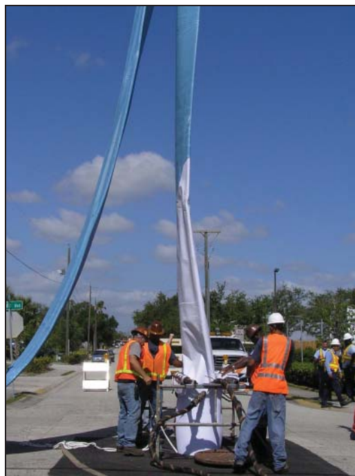
Insituform workers feed the liner into the pipe at a recent job on Apollo Boulevard, south of Hibiscus Boulevard.
