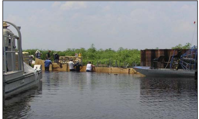
Workers with the St. Johns River Water Management District work on temporary fix to the embankment.
