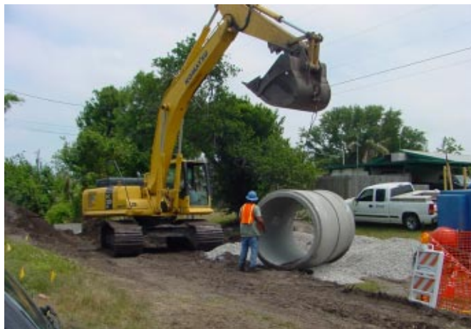
Work is underway to construct the concrete head wall to prevent erosion and stabilize the bank around the pipe.
