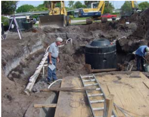
Construction Inspector Dave White observes the progress of new Lift Station 15 construction.
