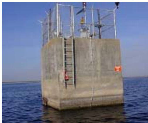
Improvements to the raw water intake structure will be the first element of the major Phase II surface water improvements project.
