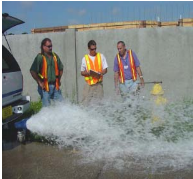
Darrell Manchester (l), environmental compliance supervisor, oversees a recent fire flow test. Matt Tanguay takes notes as Craig Silverman observes.
