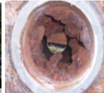
A section of old pipe from Ballard Park showing tubercular corrosion.
