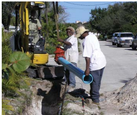
Workers with Maxwell Construction install new six-inch PVC pipe in Ballard Park.
