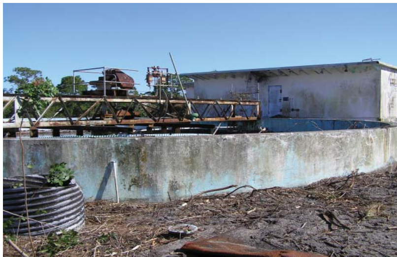
The old north plant, background, and the clarifier just prior to recent demolition.
