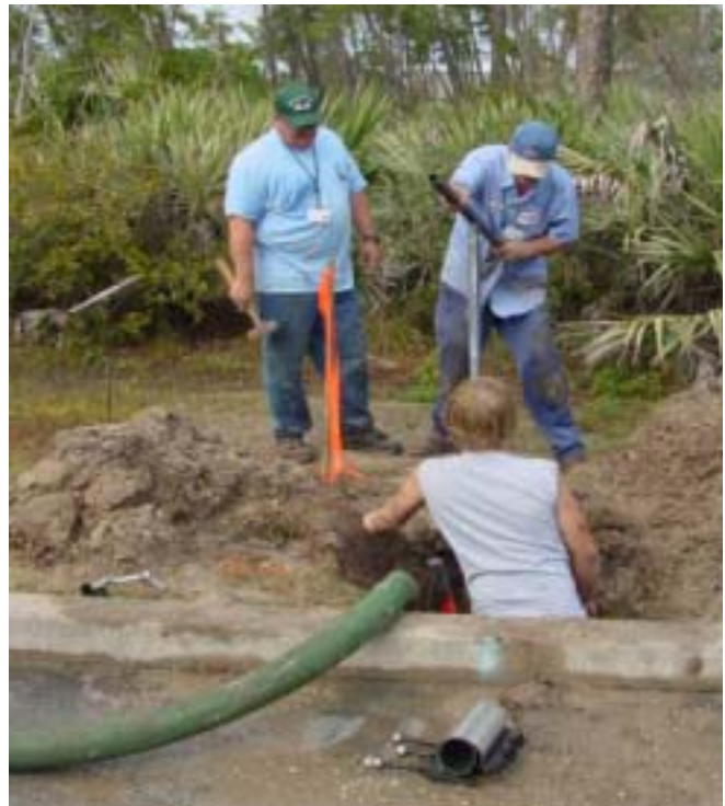
Tim Hedrick (in the hole dug to repair a water line break that recently occurred behind the Shoppes of Hidden Harbour) works on the repair. Robert Degiovine turns the valve key as Bernie Neanover stands ready to assist.
