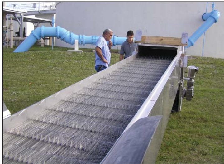
Jay Conroy (right), President of Hydro-Dyne Engineering, discusses the new influent screen with Leonard Concepcion, Wastewater Treatment Mechanic. The unit is on-site at the Grant Street Wastewater Treatment Plant being readied for installation.
