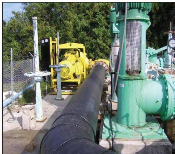
The temporary pump is the yellow unit, shown in the background.
