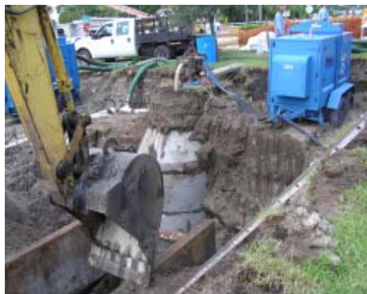
The backhoe digs down 20 feet, next to the exposed manhole, to the pipe needing replacement. The blue pumps are used to keep the hole dry by pumping out groundwater.
