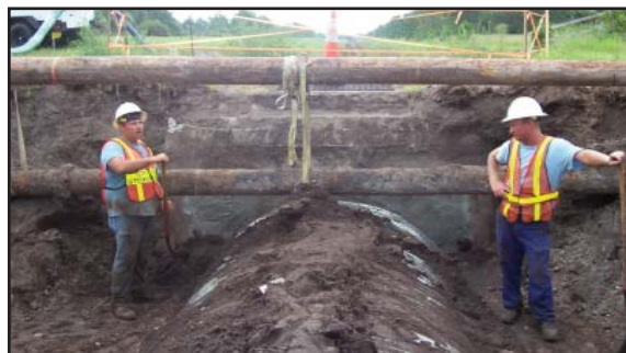
Dave Riley and Gator Hembree bring dirt to grade to prepare for paving following pipe installation. Involved also were Foreman Joe Gervais, along with Joel Mendola, Troy Parsons, Brian Harrison, Matt Carter, Josh Murwin, Silas Scott, and John Clark.
