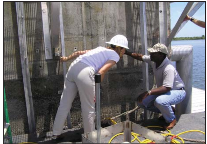
Assistant City Engineer Martha Campbell, who is project manager for the Phase II project, examines the work taking place at the intake structure, along with Water Production Superintendent Fred Davis.
