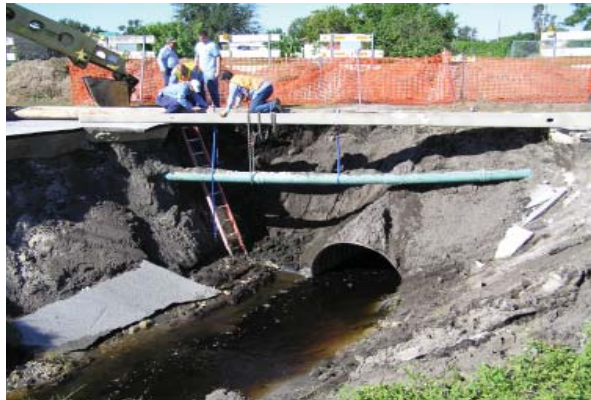
A few days after Hurricane Wilma struck, crews from both Streets & Stormwater Management and Wastewater Collections worked together to temporarily attach a sewer pipe to a pole. This was used to hold it in place until repairs could be made to the broken stormwater pipe below it.
