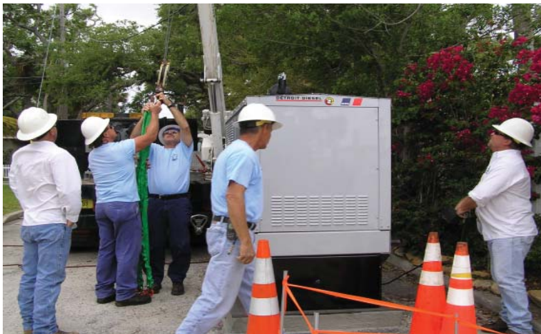
Electrician Kevin Burns, in white shirt on left, observes placement of a generator on Young Street. Shane Jones and John Taormina remove boom cords while Matt Burgeson and Wayne Noll prepare for installation. Oscar Vega also participated in the generator project.
