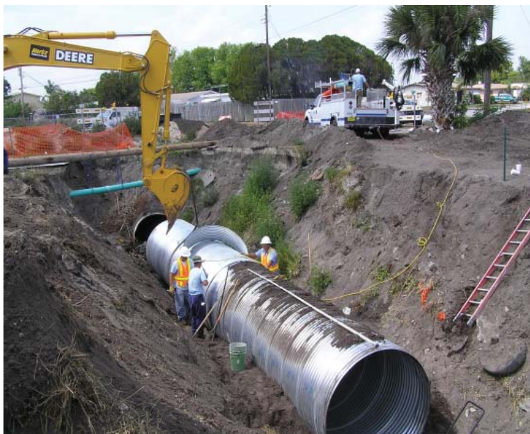
Crews from the Streets & Stormwater Division shown working on the new pipe installation.
