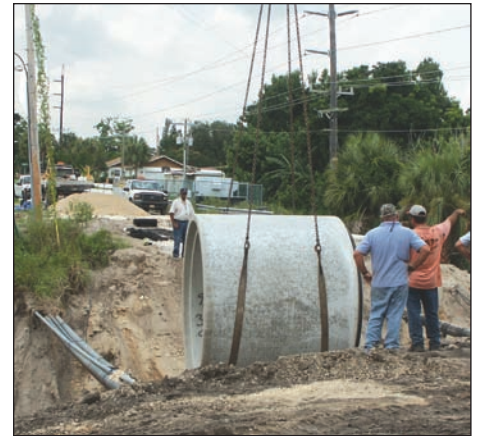
REPLACEMENT of a culvert beneath Laurie Street was among projects correcting hurricane damage caused in the last two years.
