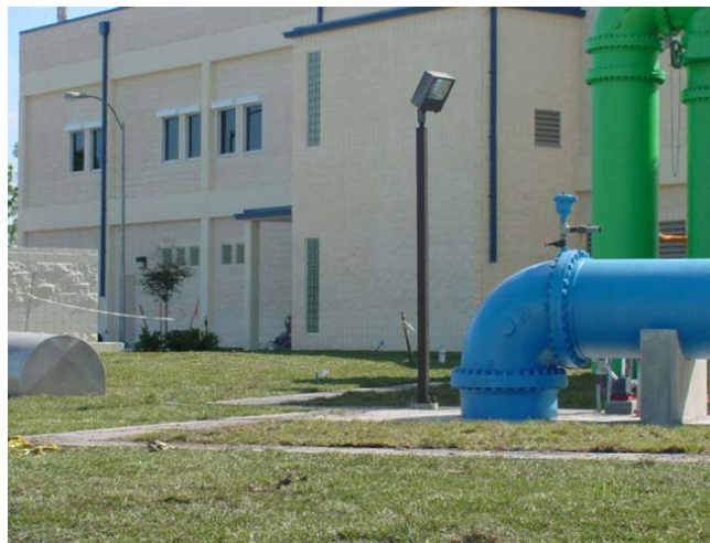
The operations building of the new surface water treatment plant is shown to the left. Water treated at this plant is obtained from Lake Washington. The green pipe is for raw water, while the blue pipe is for finished water.
